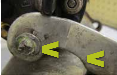
Improperly installed motor strap
