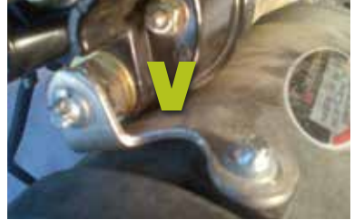
Properly installed motor strap
