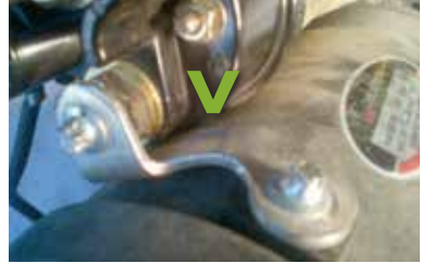
Properly installed motor strap
