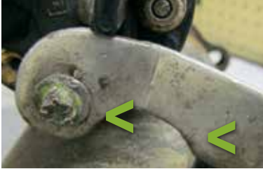
Improperly installed motor strap
