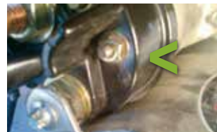
Good terminal with factory installed back up nut in place
